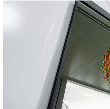
Battery cabinet.Lithium battery storage cabinet.battery ...
